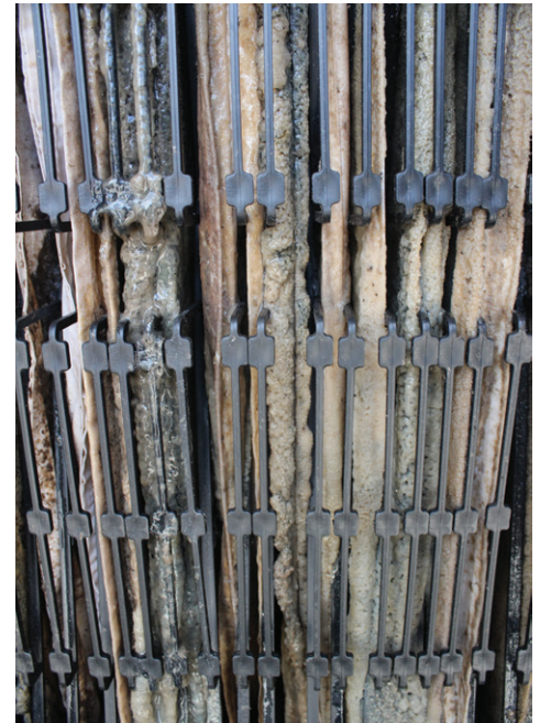
Suspended biomass vertically supported and surrounded by oxygen – a key feature of the BioGill technology.
